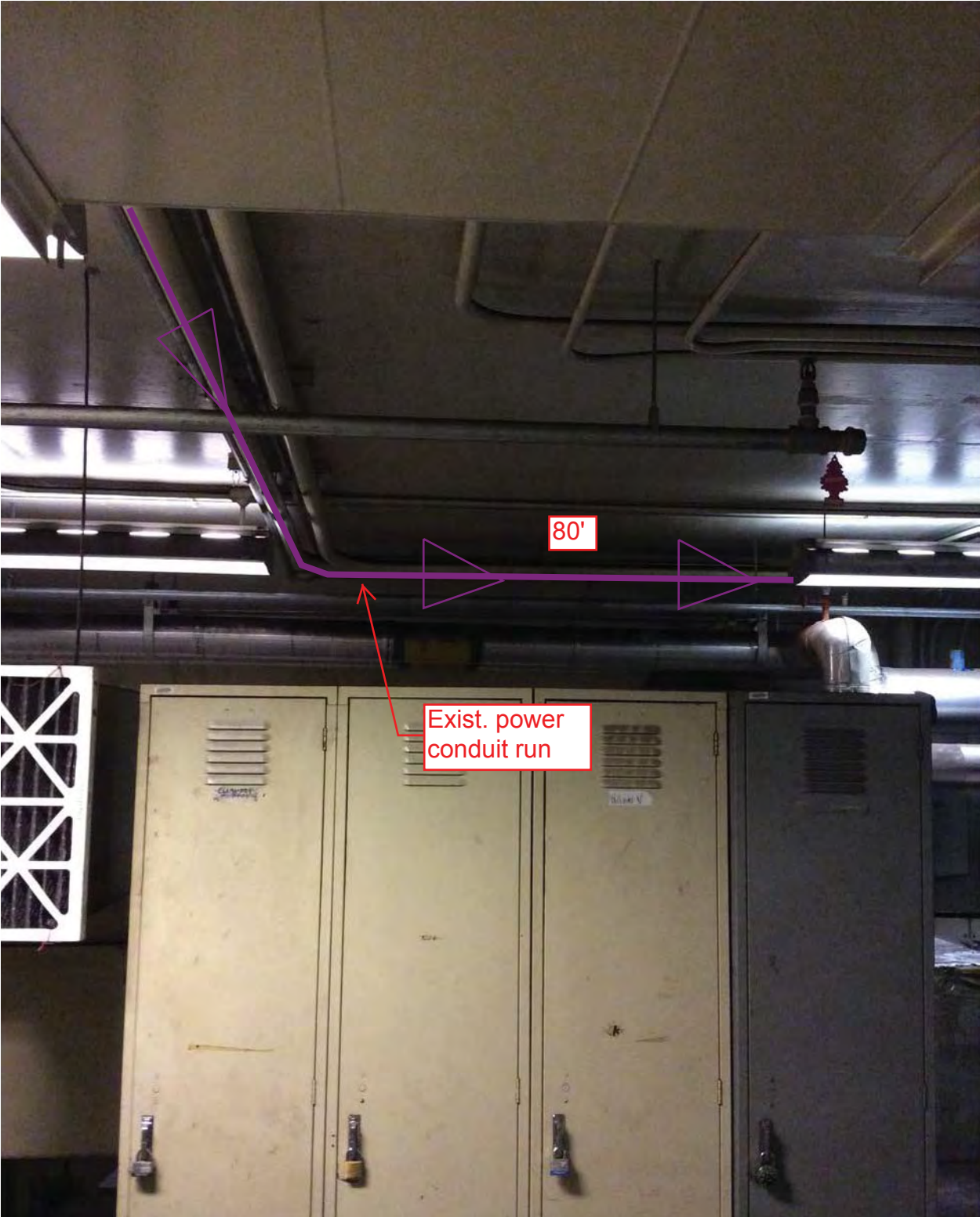
Picture 11: D07 Potomac Ave – Existing conduit from junction box 2 toward AFC Panel
