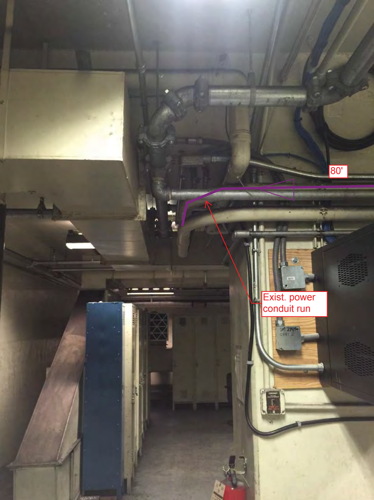
Picture 10: D07 Potomac Ave – Existing conduit from junction box 2 toward AFC Panel
